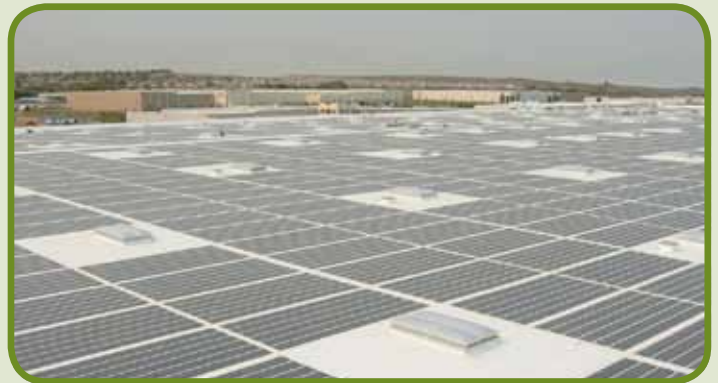
Our distribution center has one of the largest roof-mounted solar installations in California.
